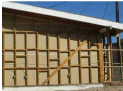
Fig. 10: Open-cell foam insulation
