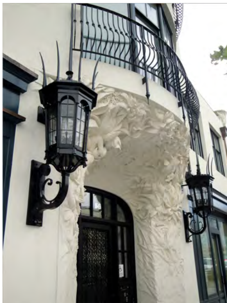
EIFS substrates can receive ornate treatments. PHOTO COURTESY OF DRYVIT SYSTEMS INC. AND EIMA
